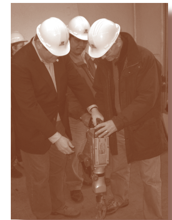
Mayor Greg Nickels (left) and Audubon President John Flicker (right) get instructions in using the jackhammer from Parks employee Sonny Gloria (center) as they prepare for the ceremonial start to renovation.
